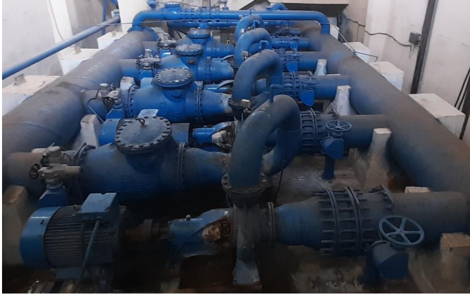
Figure 8. Water and sewage parallel electropumps.
